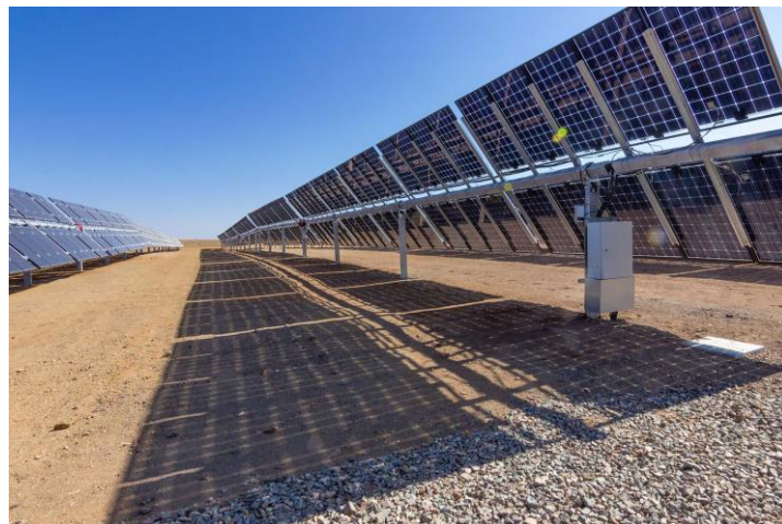
Fig.4. Solar panel array with bifacial technology
